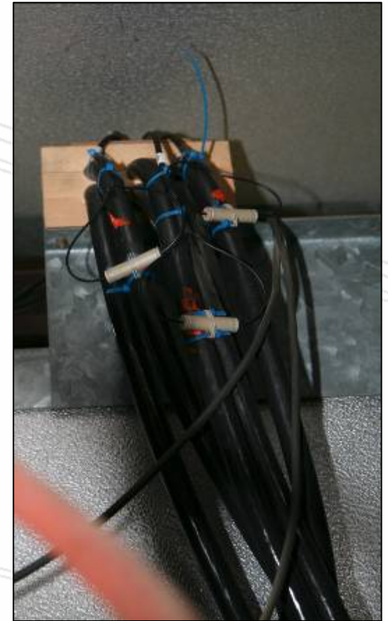
LV Transformer Cable
