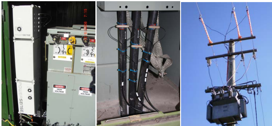
Figure 3: IED cabinet mounted in a kiosk substation, MV cable and overhead optical sensors
