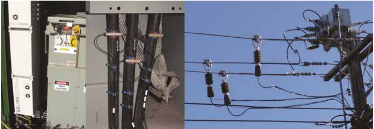
Figure 3: IED cabinet mounted in a kiosk substation, HV cable and overhead optical sensors.
